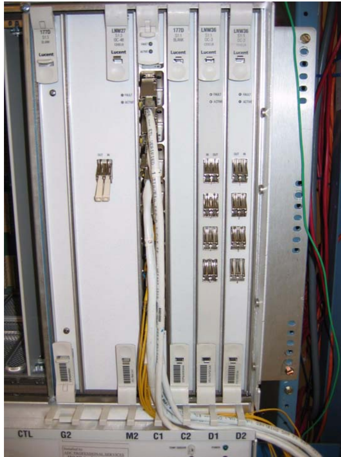
Figure 3-9 Ethernet cable routing to faceplate SFP modules
